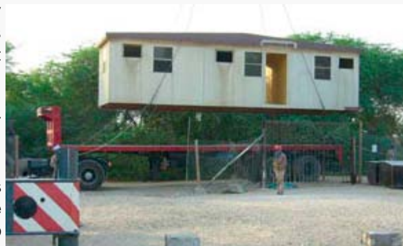
A part of the new portacabin units, donated by Gulf Contracting Company, being installed at QAWS
